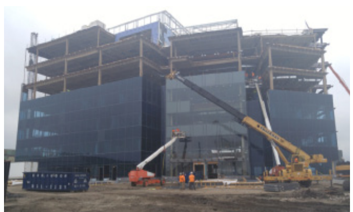
During construction, Holtec's General Contractor hired Camden residents and contracted with local companies for various aspects of the construction process.
